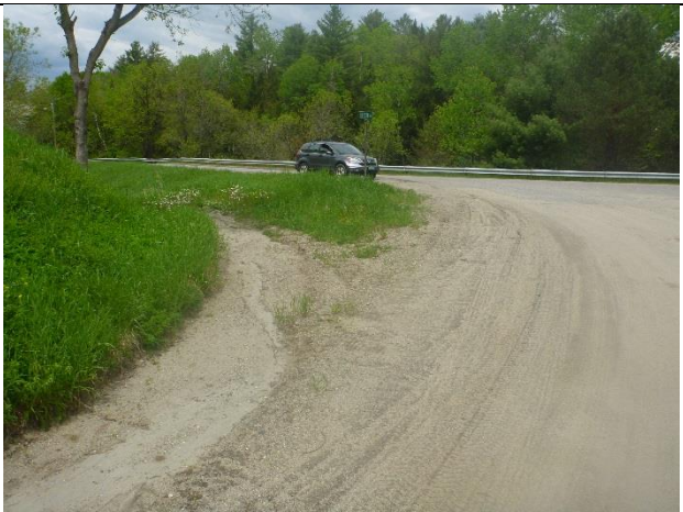
Photo 1: Ditch at the top of Tute Hill Road filled with sediment
