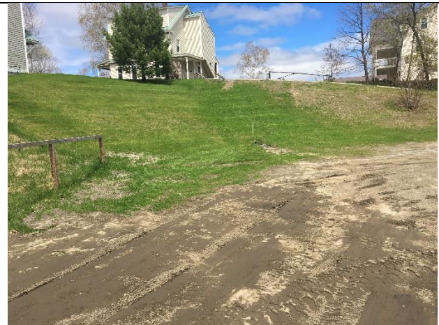
Photo 2: Erosion from the stormwater pipe across the gravel parking area.
