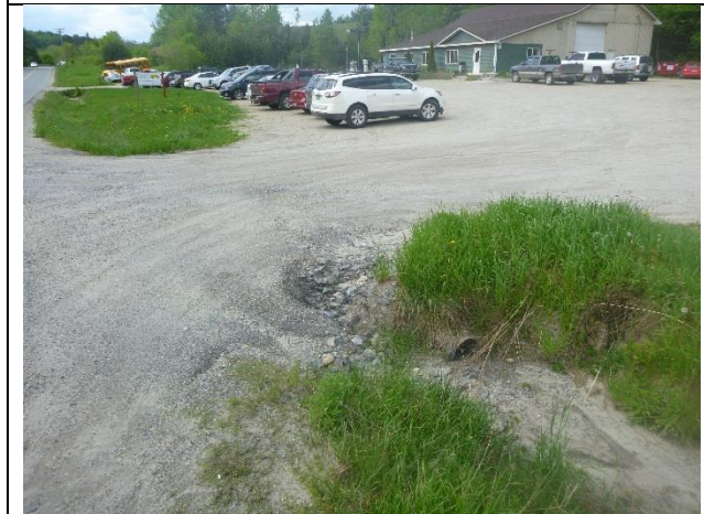
Photo 1: Gully erosion and significant sediment loading at the east entrance.
