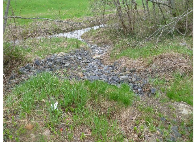
Photo 2: Armored swale that does not receive significant runoff due to parking lot grading.
