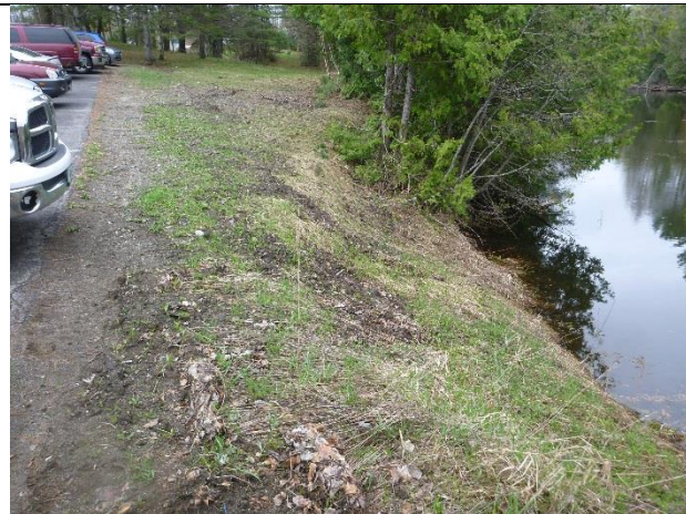
Photo 1: Erosion along the edge of pavement and the steep bank leading to the pond.
