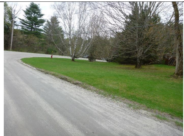
Photo 1: Poorly defined ditch spills across road causing rilling.
