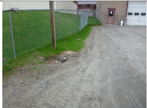
Photo 2: Erosion along edge of unpaved parking area flowing in to the catchbasin
