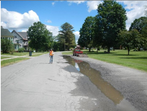
Photo 1: Low point between road and gravel parking area conveys runoff to the south.
