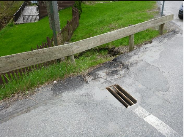
Photo 2: Evidence of recent pavement repairs and drainage point off of the road.
