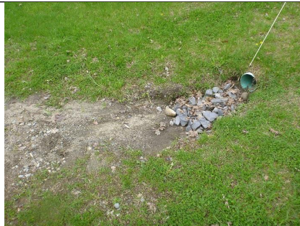
Photo 1: Erosion at the pipe outlet
