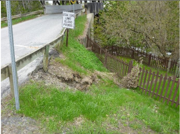
Photo 1: Gully erosion through embankment and yard to Wheelock Brook.
