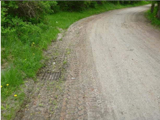
Photo 1: No ditch along steep section of road draining to a drop inlet.
