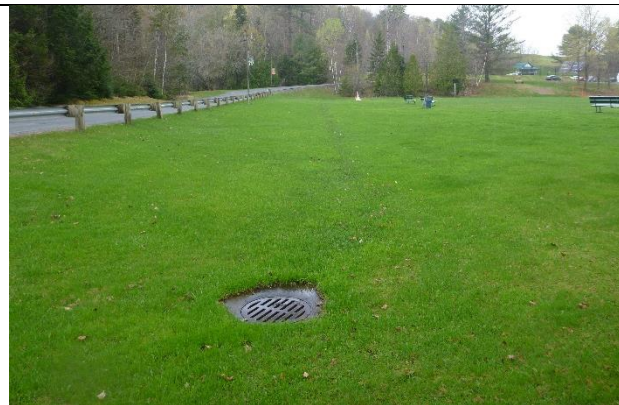
Photo 1: Mowed swale along varsity field draining to catchbasin
