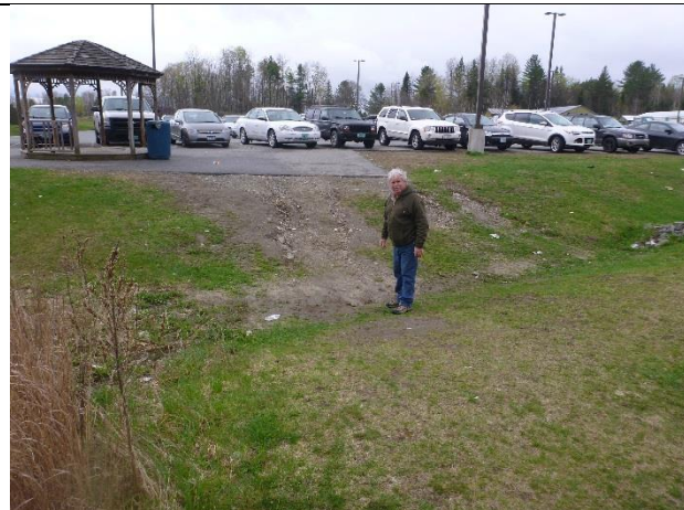
Photo 1: Erosion and compacted soils on footpath through swale at the BMP.
