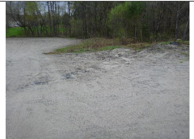
Photo 2: Water bar directs runoff from most of parking lot to a small green area on top of the slope.
