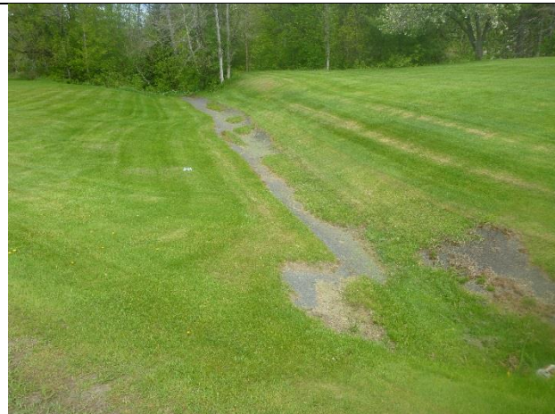
Photo 1: Asphalt ditch carrying runoff from the Lyndon Town School and Lily Pond Road.
