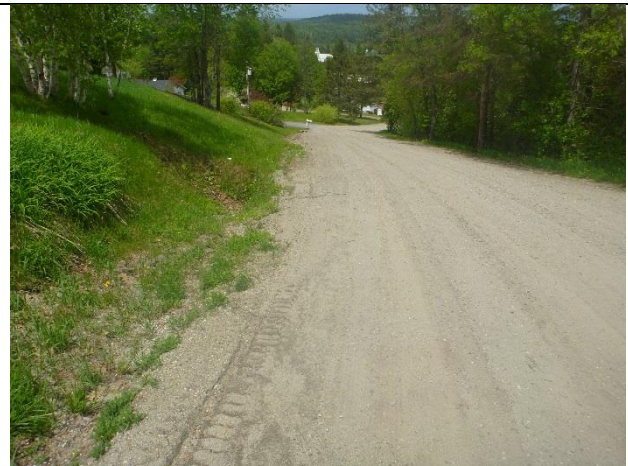
Photo 2: Steep section of road with unstable ditches.
