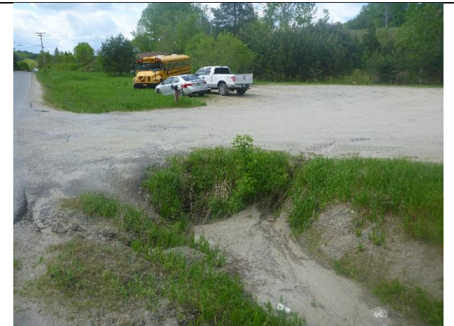
Photo 2: Gully erosion and significant sediment loading at the west entrance.
