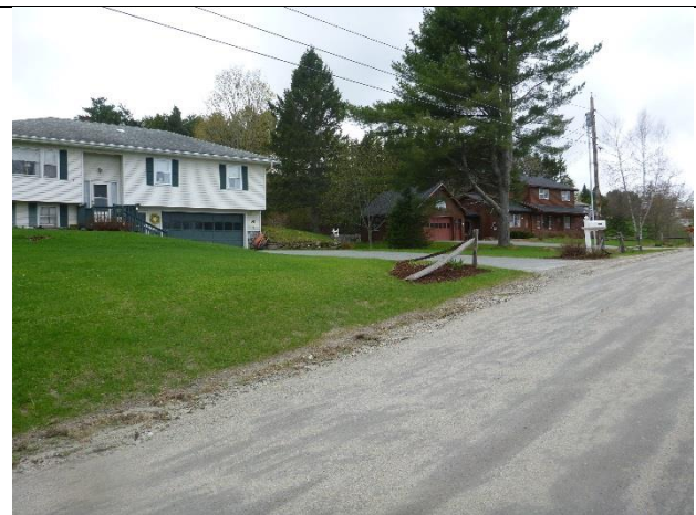
Photo 2: Erosion along road shoulder and poorly defined ditch.
