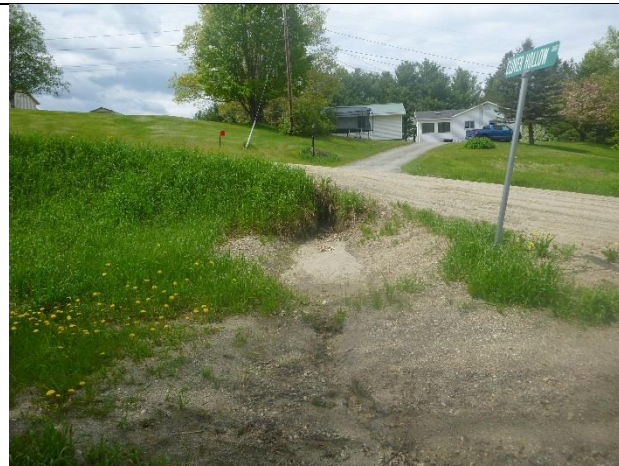
Photo 1: Large sediment deposits along Clover Hollow Rd adjacent to an intermittent stream.
