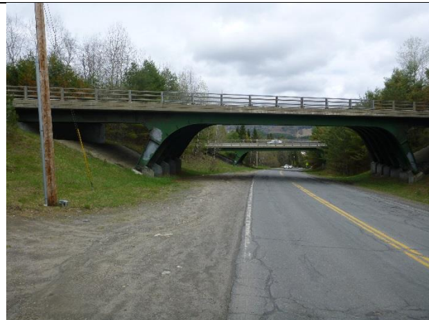
Photo 1: Poorly defined ditch with bare soil and active erosion.
