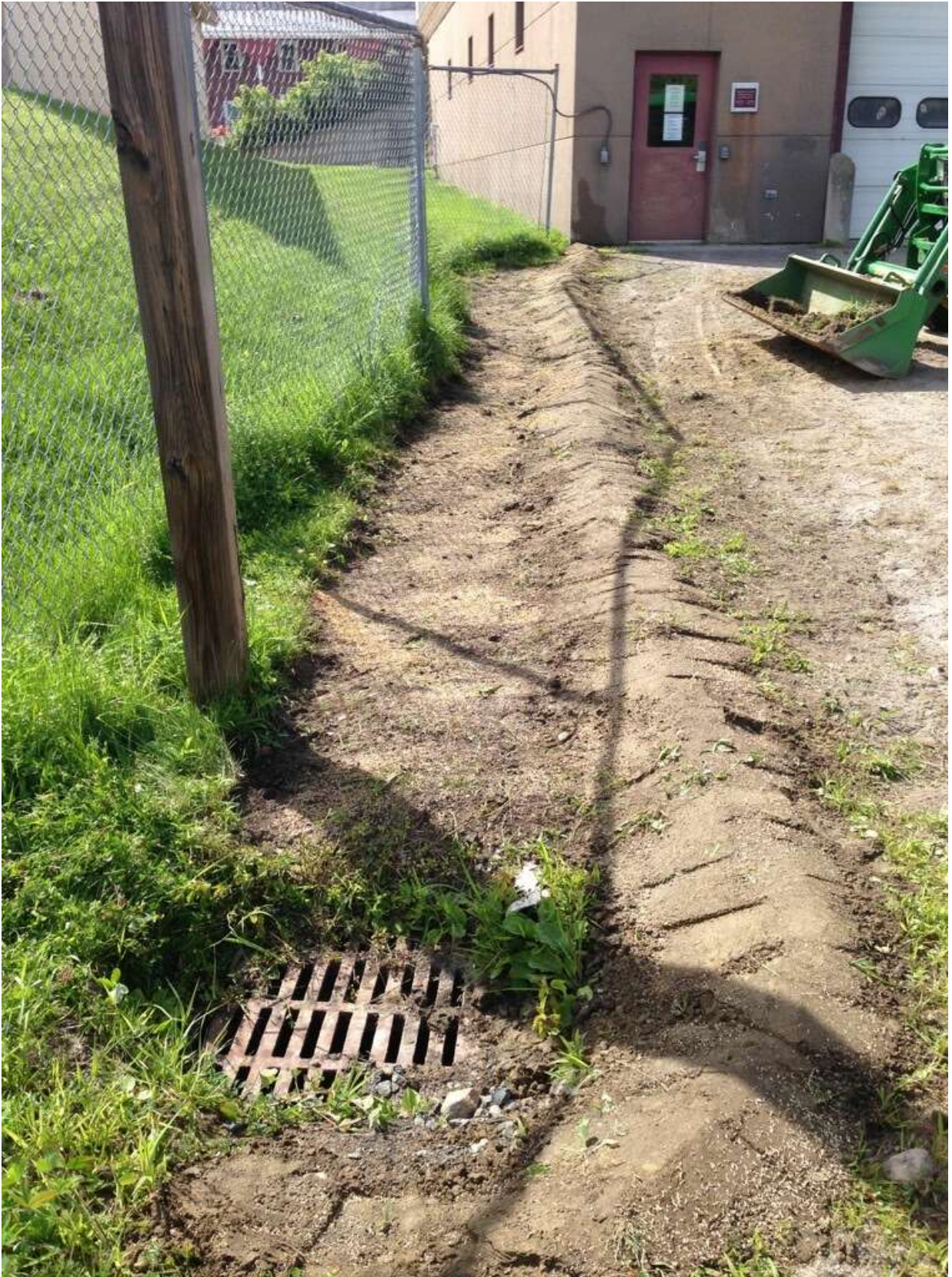
Figure 2: A small swale created to convey clean water from the rooftops to the existing catch basin.
