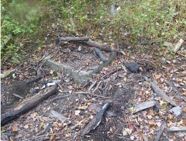
Figure 2: Existing outlet structure – two 24” square grates partially obstructed with debris
