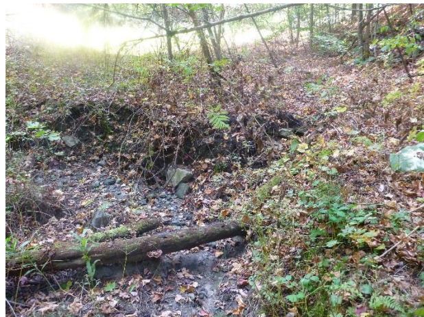
Figure 5: Active erosion in the channel carrying runoff from the Pinehurst and High St culverts
