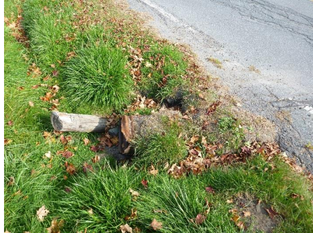
Figure 10: Erosion at the culvert inlet
