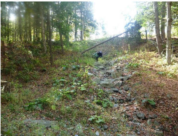
Figure 4: Heavily armored flow path from the Chase St. culvert outlet
