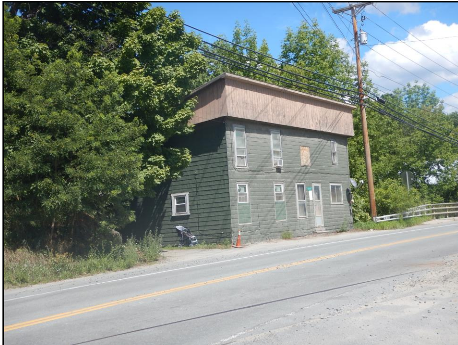
Photo 6. Photo shows a structure located on the northwest corner of the bridge spanning the Moose River. View is to the northeast.
