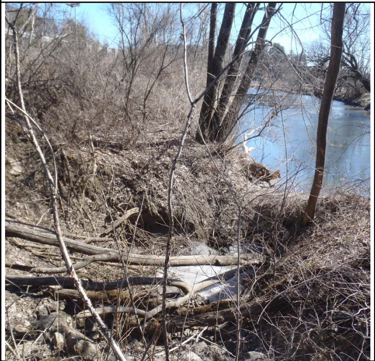
Photo 1: Scour pool at discharge point.
